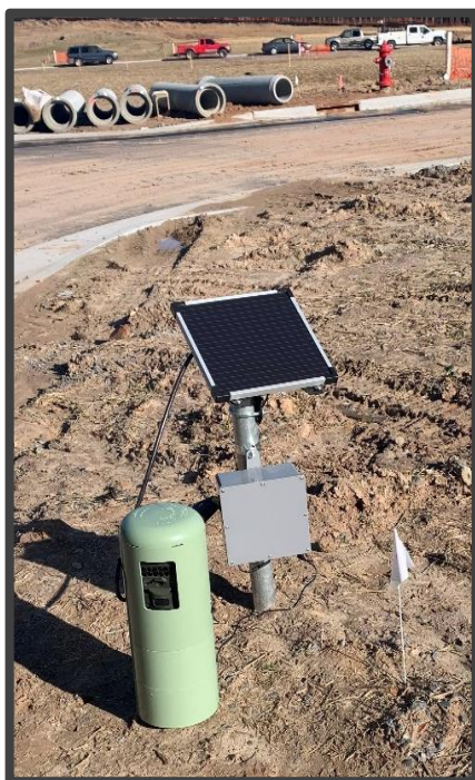
Actual installation photo of license plate reader camera on job site. Camera is mounted and concealed within pedestal.
