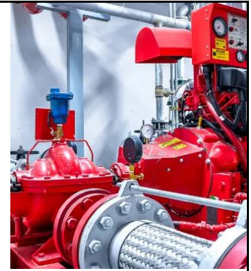
Fire Pump Feeds
